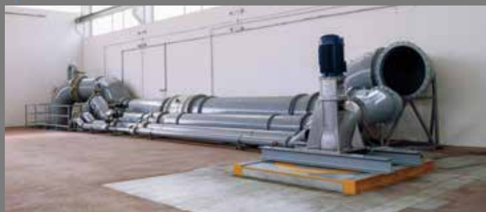
Sala prove Testing Room
